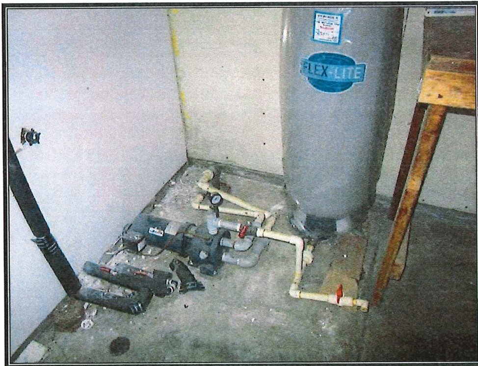
Domestic well/pump in garage reportedly not operation. (A15-123)
