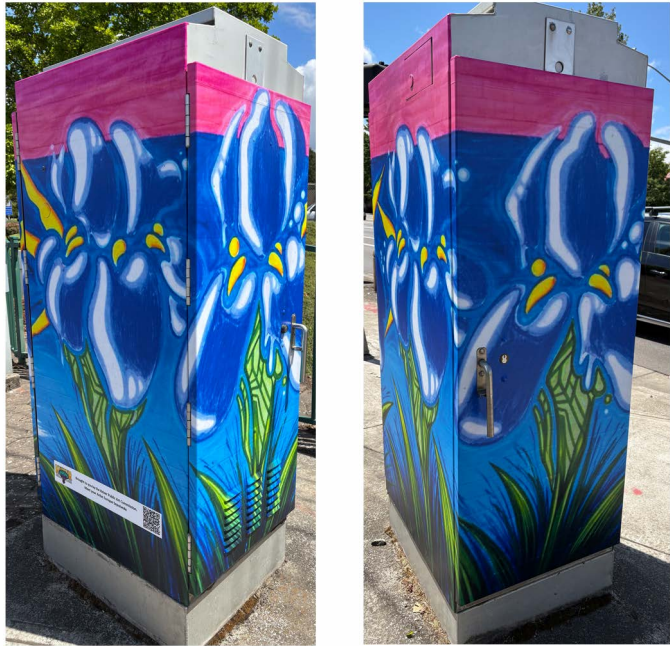
Artwork As Installed
